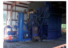
Compressor directing methane to the flare
